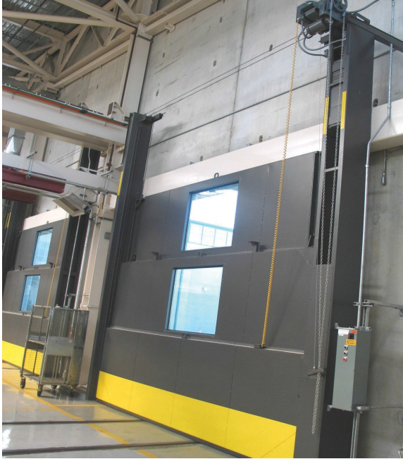
1 PSI Three Panel Vertical Lifting Fueling Door for Metro Transit System Garage
